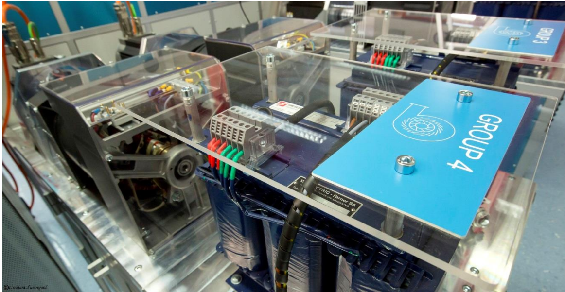
Fig. 3 – Synchronous machine and transformer of the four production groups
