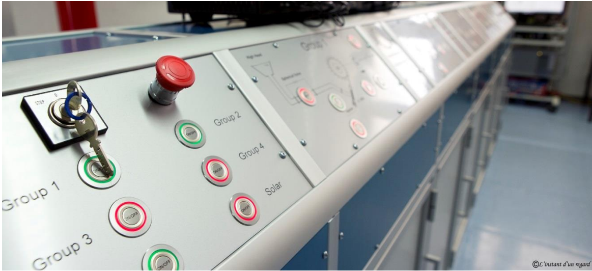
Fig. 5 – Detail of the control panel of the synchronous machines
